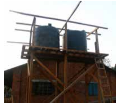
Gravity fed water cistern
